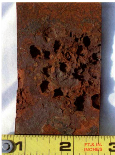
FIGURE 4 On this pipe sample, a group of deep, narrow pits were discovered at the point where they were just beginning to interconnect.
