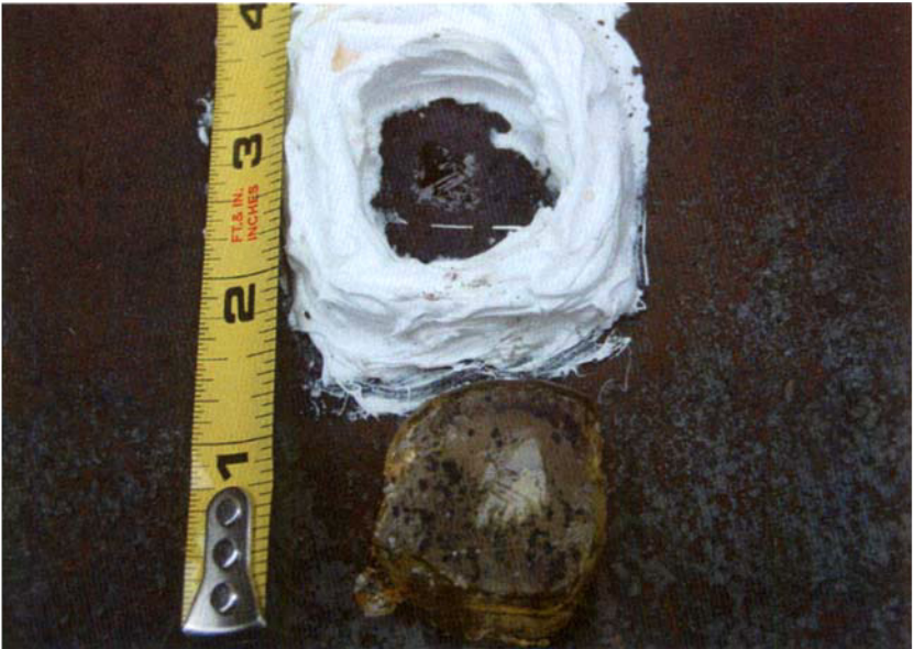
FIGURE 16 (Top) An embedment that has just been performed on a corroded pipe surface. (Bottom) embedment removed from pipe.
