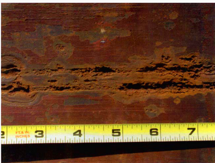
FIGURE 6 Close examination of this sample showed that narrow groups of corrosion pits occurred at damaged internal flow coating in a gas pipeline, forming long, continuous pits.
