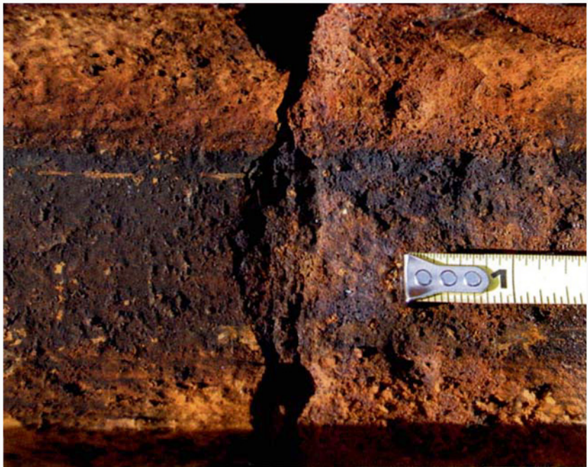
FIGURE 8 The root pass and heat affected zone of this girth weld exhibited preferential attack as compared to corrosion of the surrounding pipe metal.
