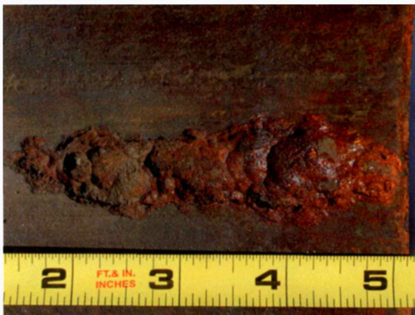
FIGURE 5 A group of larger pits have grown together to form one continuous axial pit in this pipeline sample.
