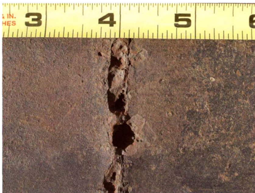
FIGURE 11 Corrosion pitting at a girth weld that was proven, through comprehensive field and laboratory testing, to have resulted primarily from microbial activity.
