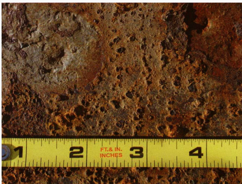
FIGURE 2 Numerous isolated pits have formed on this pipe surface beneath a semi-protective scale.
