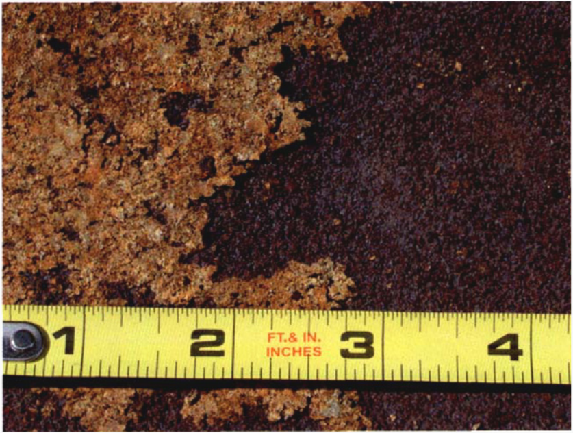
FIGURE 7 General attack of the pipe surface (at right) has occurred here beneath a thin layer of non-adherent debris (left).
